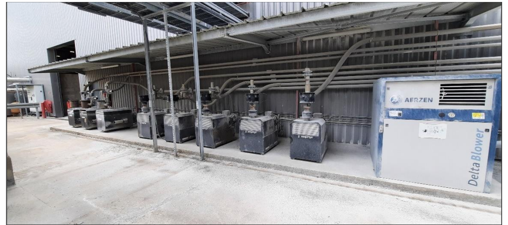
Zone turbines – Pt 22
